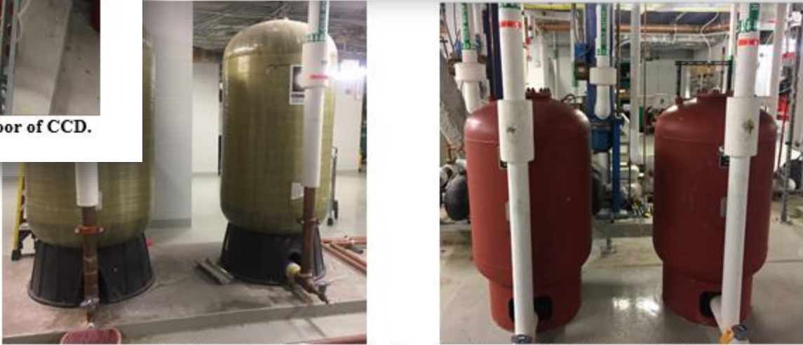
Figure 2: Bladders Cold #1 and #2 (left) and Bladders Hot #5 and #6 (right) in the CCD Penthouse.
