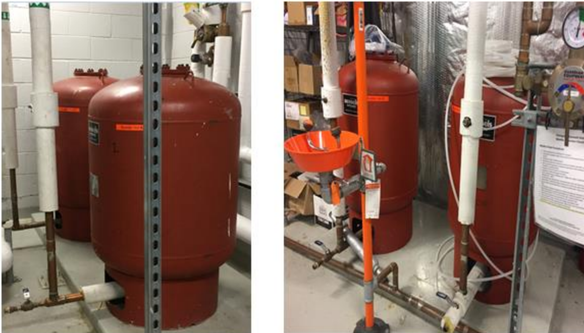
Figure 1: Bladders Hot #1 and #2 (left) and Bladders Hot #3 and #4 (right) on the 2nd floor of CCD.
